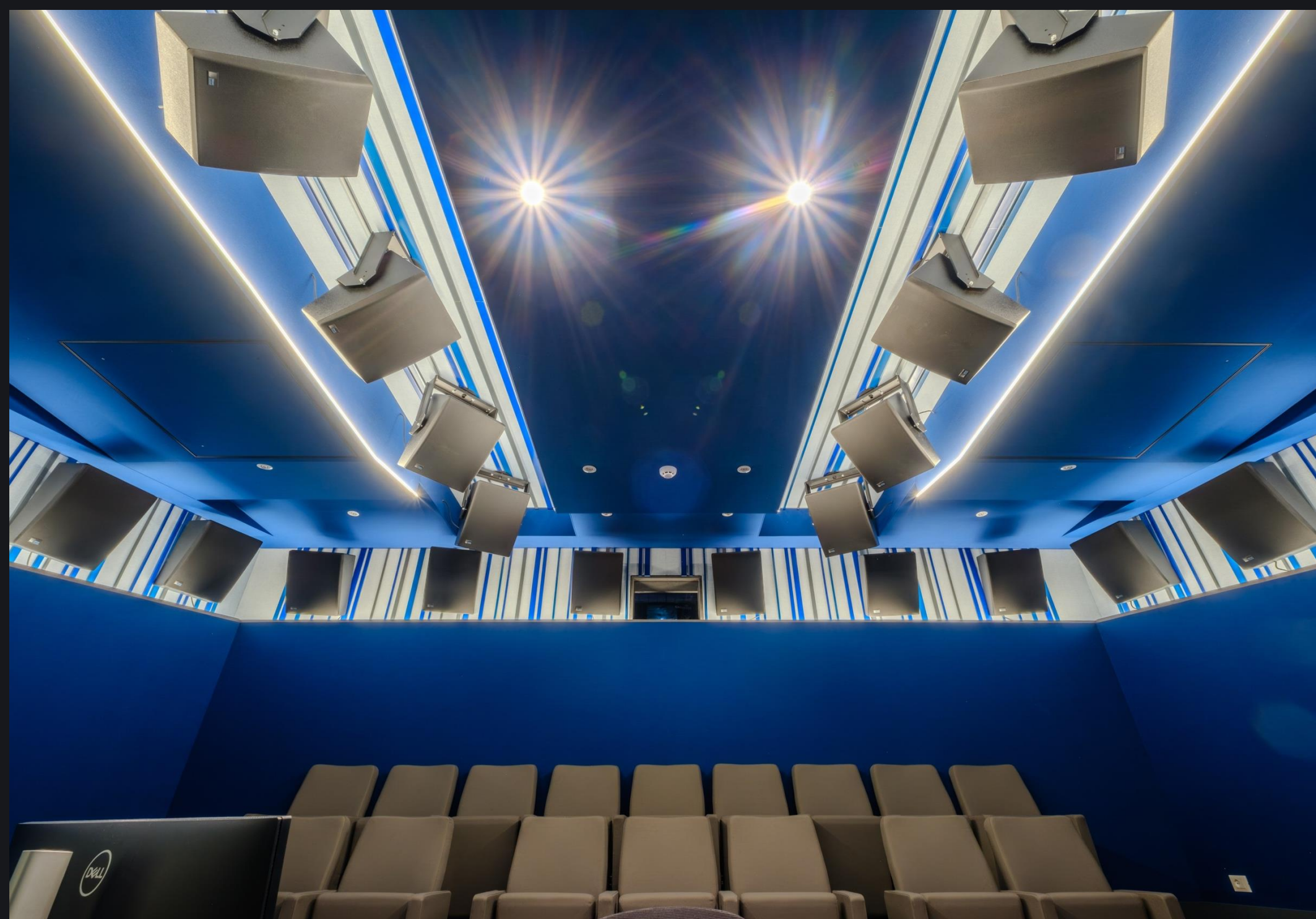
The Atmos ceiling of the theatrical room.
